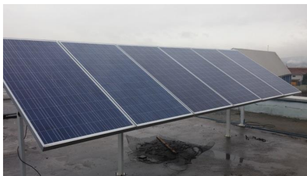
Fig.1: The installed PV system
